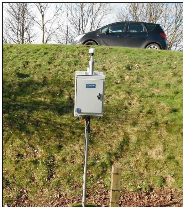
Figure 2: Example of an installed Automatic Light Scatter Dust Meter
