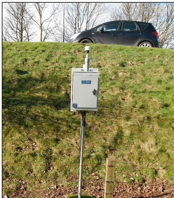
Figure 2: Example of an installed Automatic Light Scatter Dust Meter
