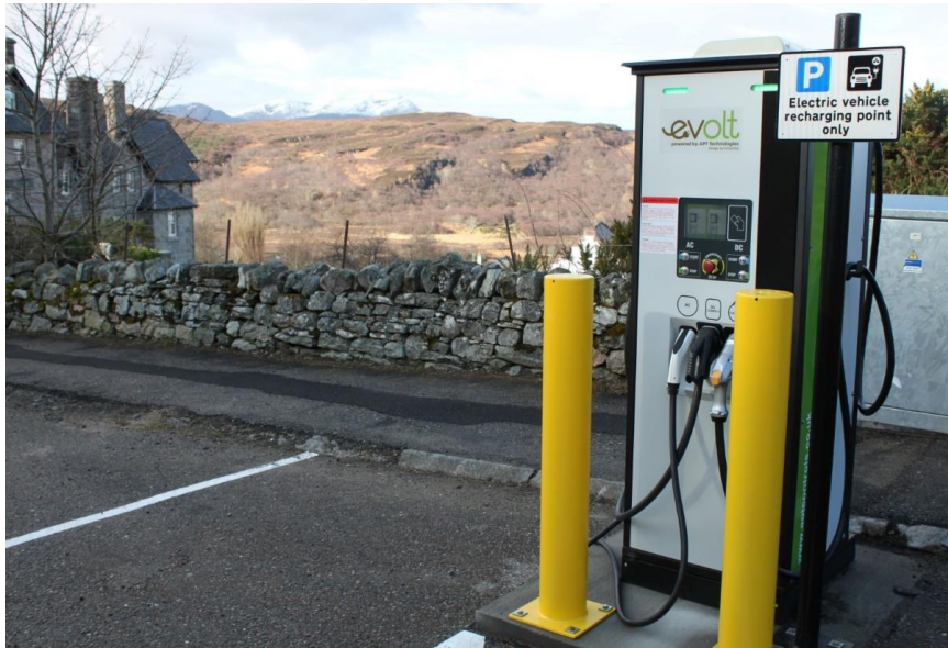
Figure 10 – 50 kW Rapid Charge Point in the Highlands offering AC Type 2, DC CCS (COMBO 2) and DC CHAdeMO connectors (Source: Urban Foresight)
