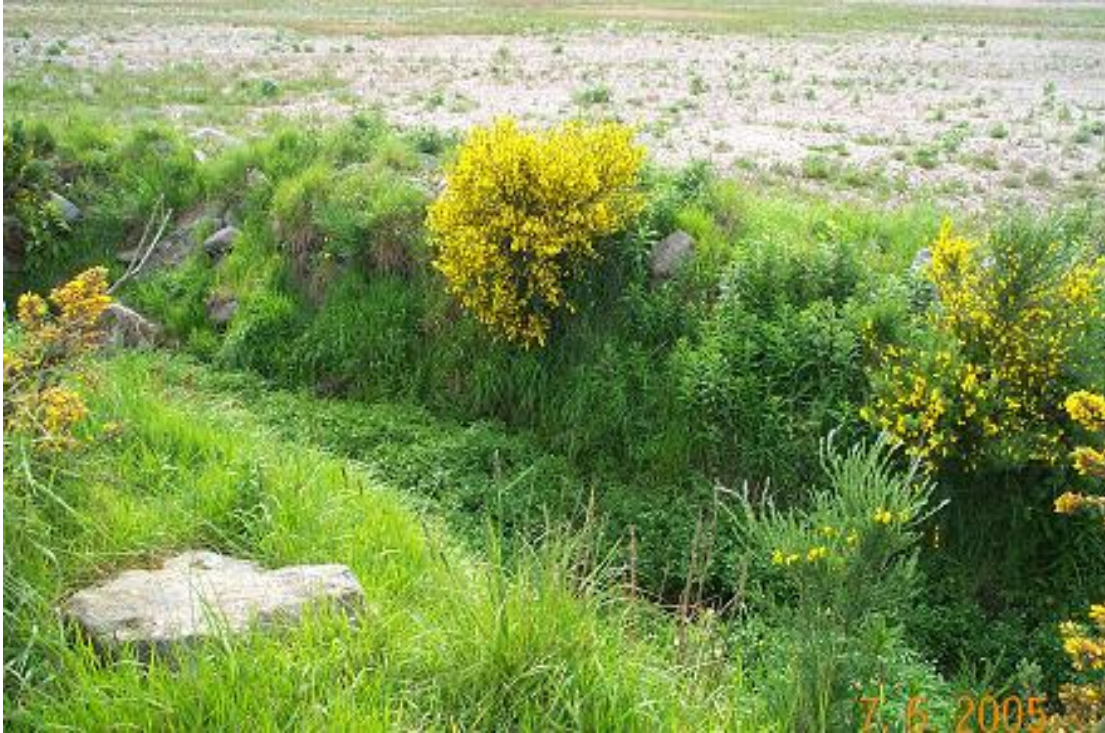
View looking downstream of the channel of the Red Moss Burn at the location of the proposed road crossing. The channel shows evidence of past straightening, widening and deepening. The bed of the channel is obscured by dense vegetation which has grown on silt deposits within the channel.
