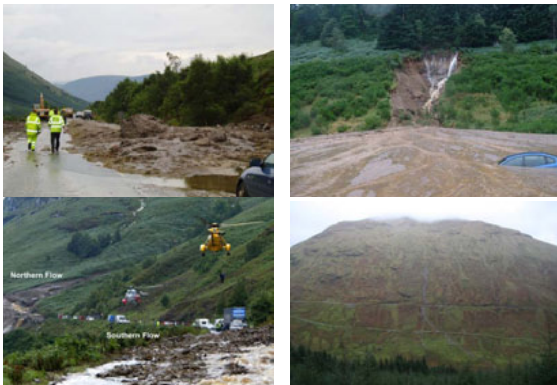
Examples of landslides affecting the Scottish trunk road network. Top left: A83 Cairndow, August 2004. Top right: A9 North of Dunkeld, August 2004. Bottom left: A85 Glen Ogle, August 2004. Bottom right: A83 approach to Rest and be Thankful, October 2007.
