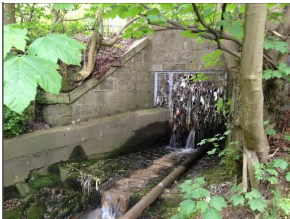
a) Upstream view of Scatter Burn downstream of the railway culvert. Note: trash screen partially blocked with debris.
