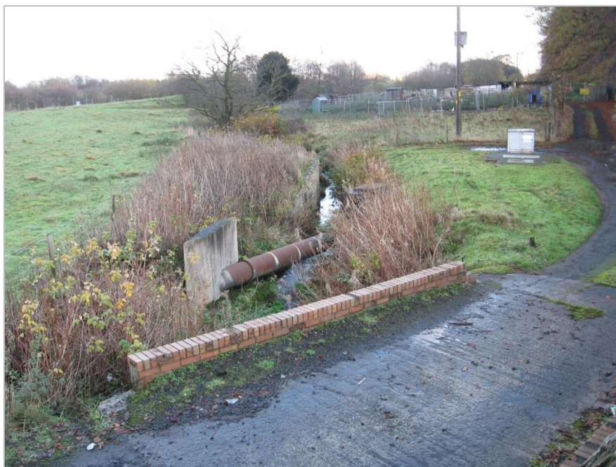
Plate 5.8 - Foul Drainage Pipe Crossing the Dean Burn at the Pumping Station and Behind, Surface Water Drainage Outfall from a Section of the A720
