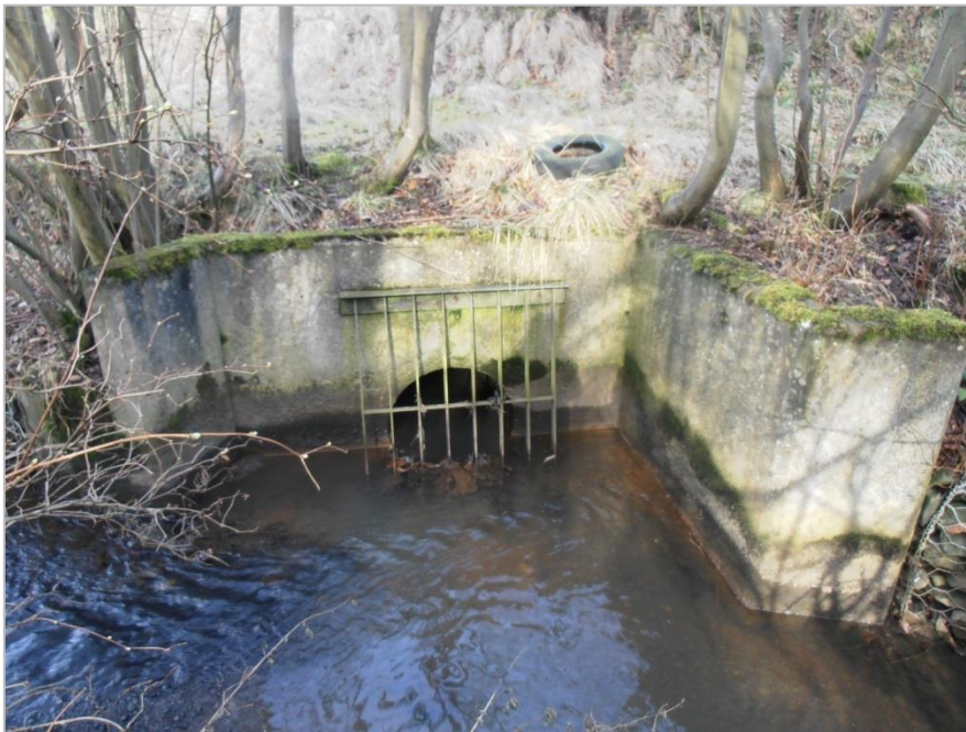
Plate 5.3 - Dean Burn at the Surface Water outflow Downstream of the Pumping Station
