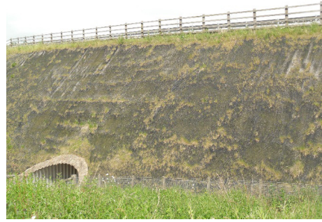
Figure 4: Failed regeneration/unsuccesful planting around culvert
