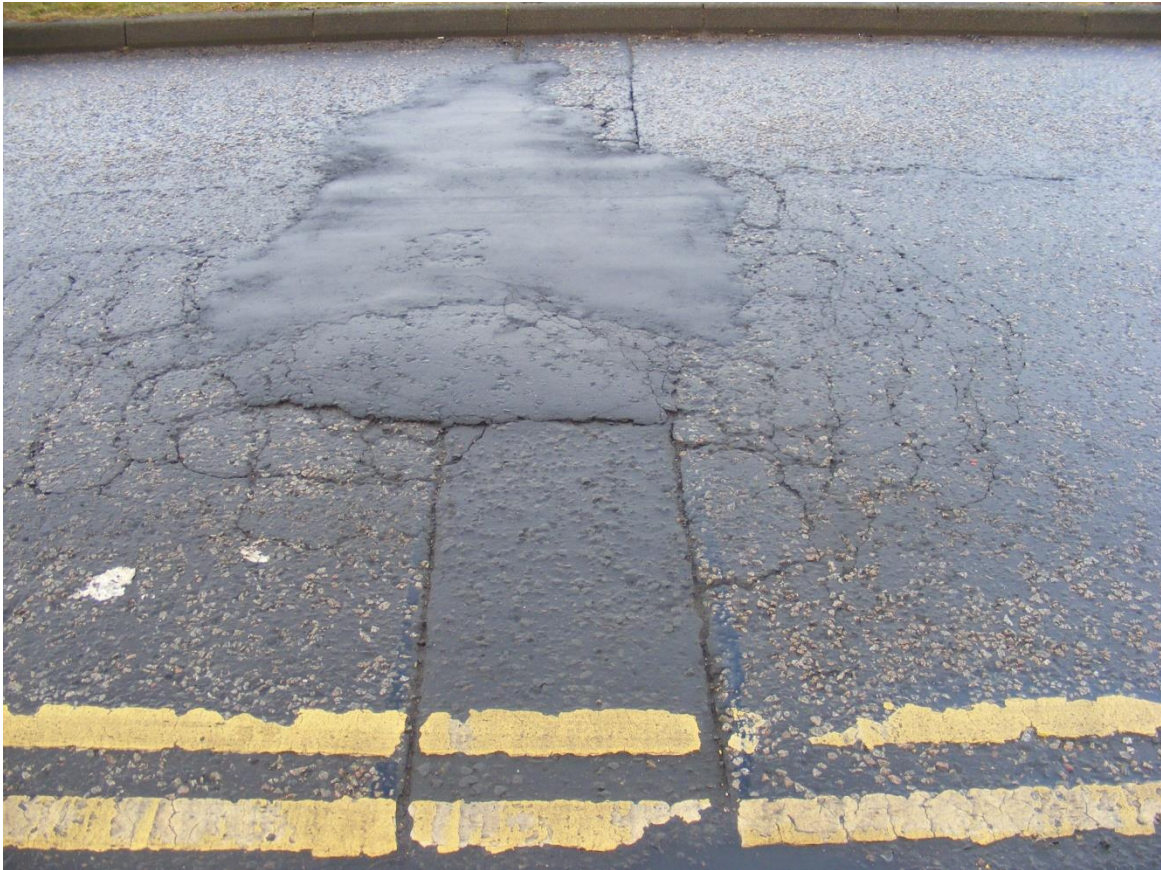
Figure 3 – example of a reinstatement which appears to be having an effect on the surrounding carriageway
