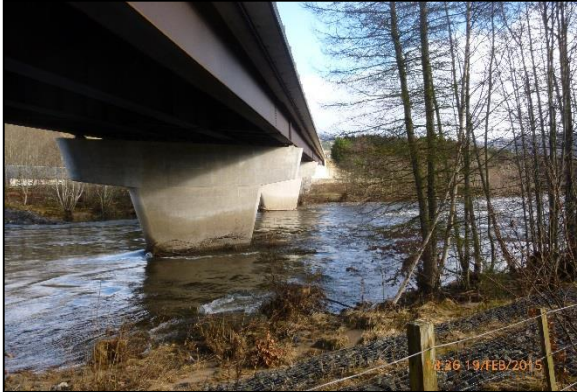
Existing Essangal Underbridge looking over to eastern bank of the River Garry
