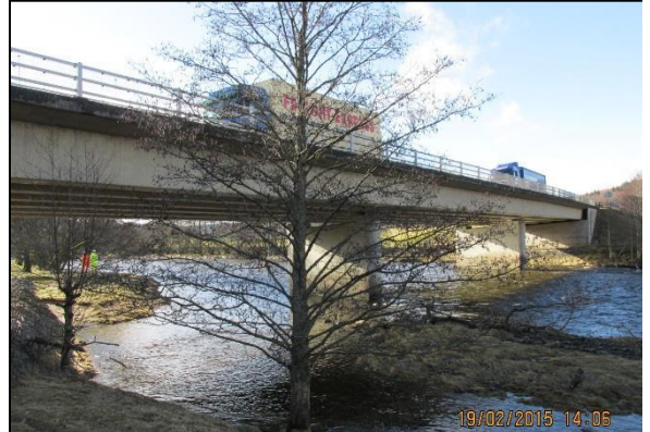
Existing Pitaldonich Underbridge crossing looking over to eastern bank of the River Garry
