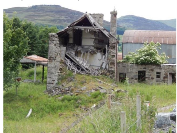
Photograph 2: Collapsed gable end
