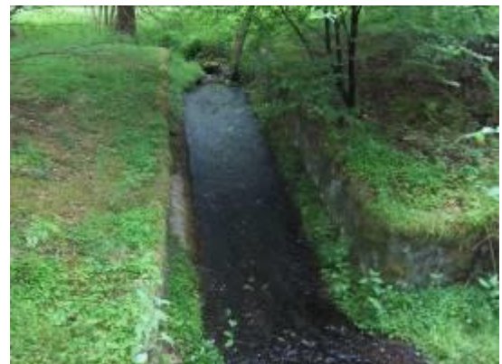
Photograph 12: View of WF69 immediately upstream of existing A9 culvert and confluence with additional channels (straightened planform).
