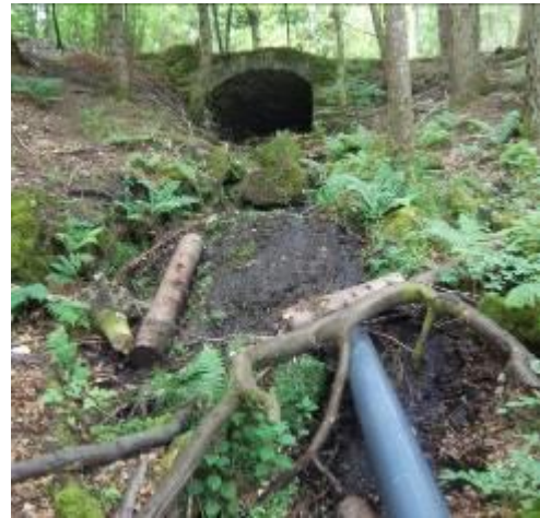
Photograph 16: Upstream view of WF76 immediately downstream of General Wade's Military Road culvert.
