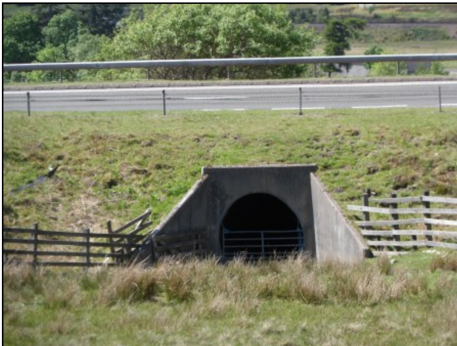
Photograph 8-3: Existing sheep creep at ch. 22,750
