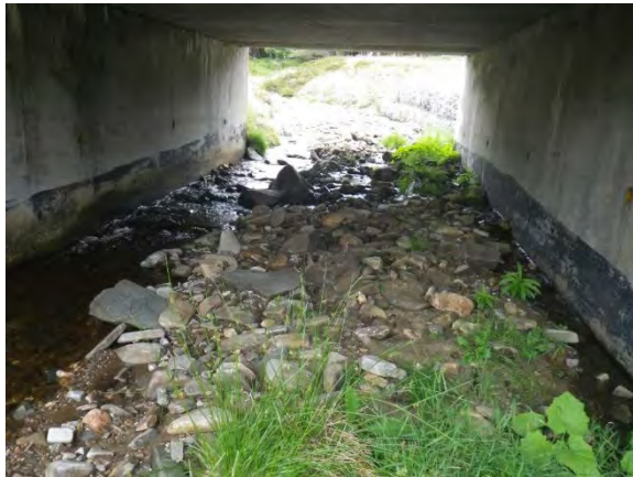
Photograph 11.4.3.33 - Deposition in A9 crossing, creating low flow channel
