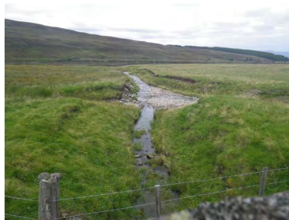
Photograph 11.4.3.9- Downstream to confluence with crossing 64, failing channel banks
