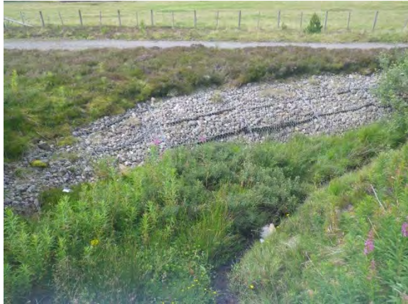
Photograph 11.4.3.21 – Gabions on left bank of channel have been undercut. Channel is undersized for high flows
