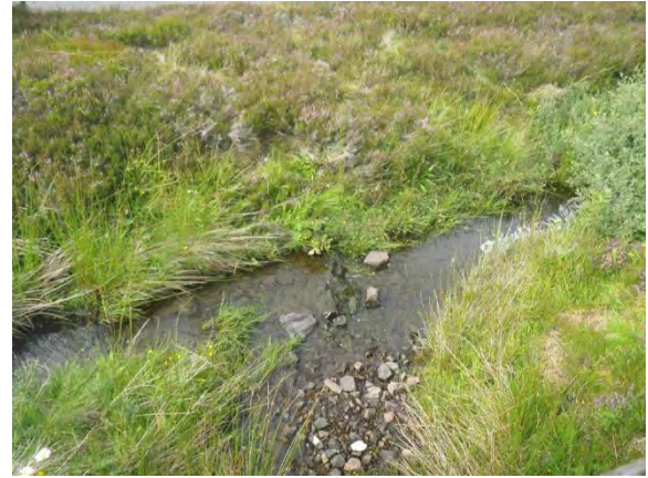
Photograph 11.4.3.23 – Erosion of concrete slabs in bed of drainage channel. High energy system despite lower bed slope than upstream channels
