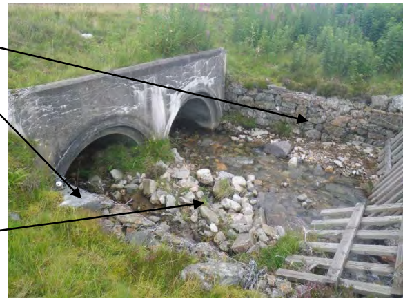
11.4.3.14 - Deposition of coarse material in culvert entrance
