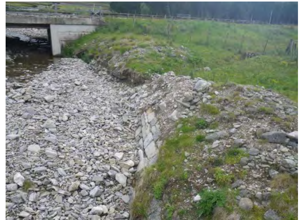
Photograph 11.4.3.2- Erosion of right bank
