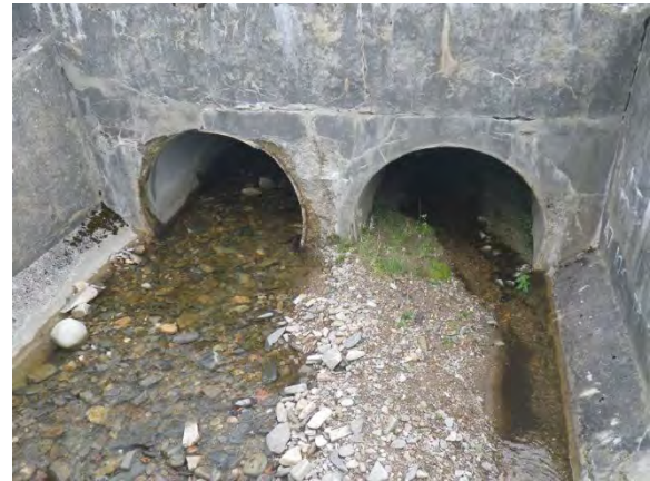
Photograph 11.4.3.12- Deposition in both pipes downstream of crossing
