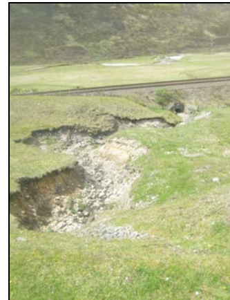
b) Downstream view west of A9 showing evidence of incision
