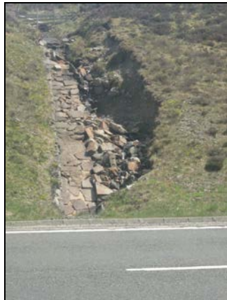
a) Upstream view of damage to bed armouring east of A9
