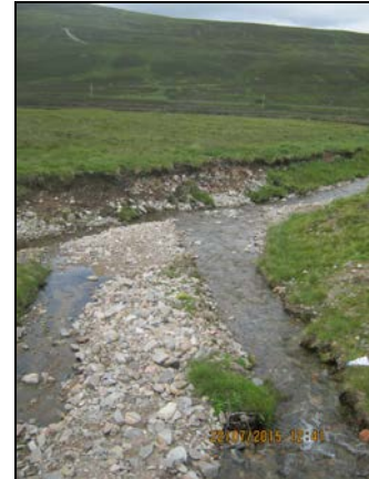
b) Downstream view west of A9, showing bank collapse and a channel bar
