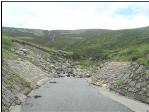
a) Upstream view east of the A9, showing bed and bank protection
