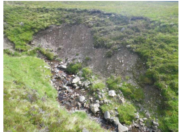
Photograph 11.4.3.33- Erosion of valley side
