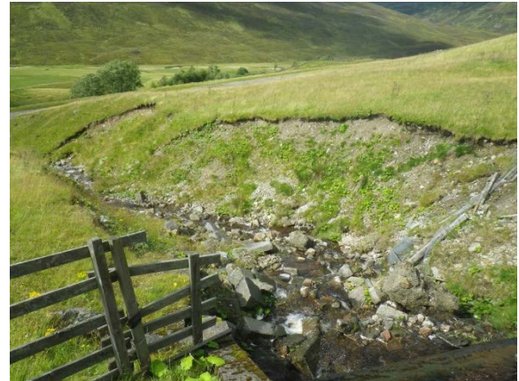
Photograph 11.4.3.27-Downstream bank instability due to channel insision
