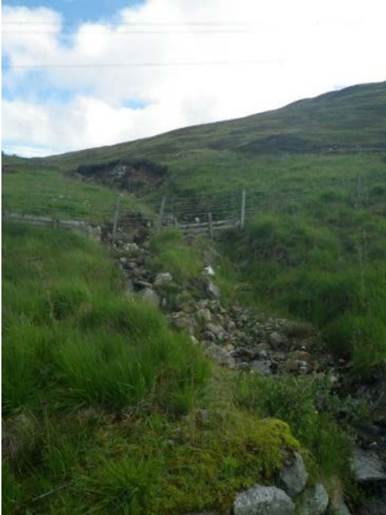
Photograph 11.4.3.1- Erosion upstream of crossing producing excess sediment
