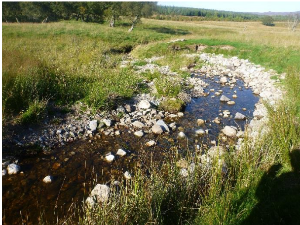
P1030909 – View immediately downstream of existing A9 culvert with unnaturally placed boulders on the outside bend (NGR NH 751 348)
