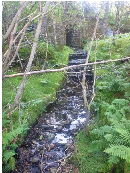
P1040028 – View from downstream towards existing railway bridge with heavily modified bed and banks (NGR NH 772 340)
