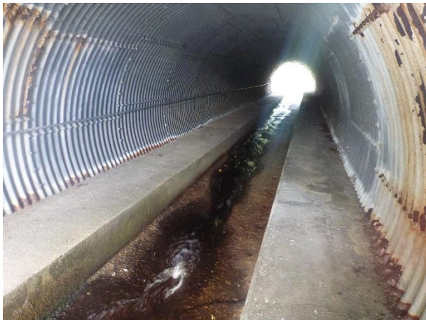
P1030789 – View downstream through existing A9 culvert showing concrete bed and banks (NGR NH 797 300)
