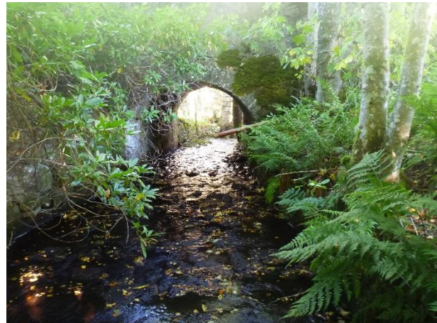
1030905 – View upstream of bank and bed protection underneath railway bridge (NGR NH 765 345)
