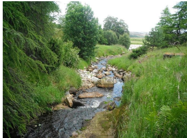
DCSF3950 – View downstream from culvert exit; the concrete apron has failed at the end of the culvert; limited gravel deposits on the left hand bank (NGR NH 797 300)
