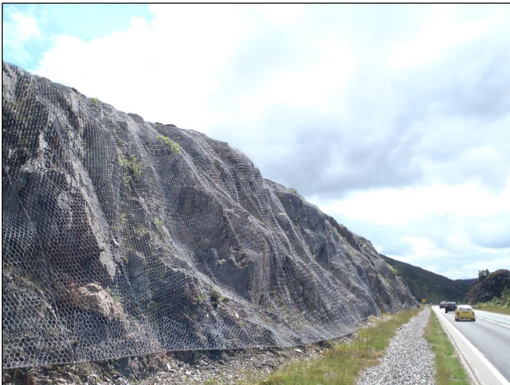
Figure 10 View southeast of the cutting at Slochd Summit with rockfall protection mesh.
