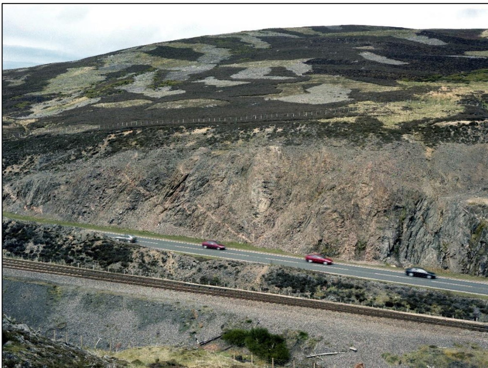
Figure 16 View to the east of the Slochd Summit rock cutting (before rockfall protection mesh installed). The Highland Main Line can be seen in the foreground. Photograph supplied to AMJV by the BGS, ©BGS
