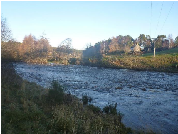
P1040617 – View immediately downstream of railway bridge, erosion (likely poaching) on the RHB (NGR 2897 8227)
