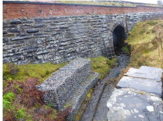
P1040970 – Channel between the railway and A9 was lined with gabion and stone wall protection through two culverts (NGR 2837 8254)
