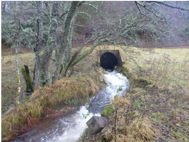
P1040532 – The channel emerges from a large culvert underneath the A9 (NGR 2867 8100)
