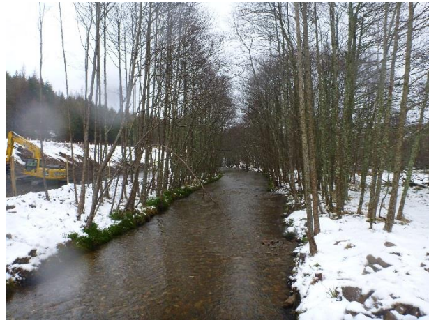
P1040417 – View downstream from temporary crossing showing wide and uniform channel leading towards Loch Alvie (NGR 2855 8092)
