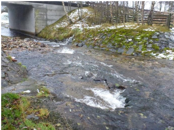
P1040468 – Collapse concrete/cobble bed leading towards the existing A9 crossing (NGR 2884 8106)
