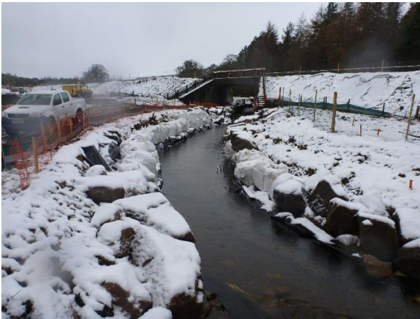
P1040416 – View upstream towards existing A9 crossing; the channel had been lined artificially with rip-rap and boulder protection as part of the ongoing construction works (NGR 2855 8092)
