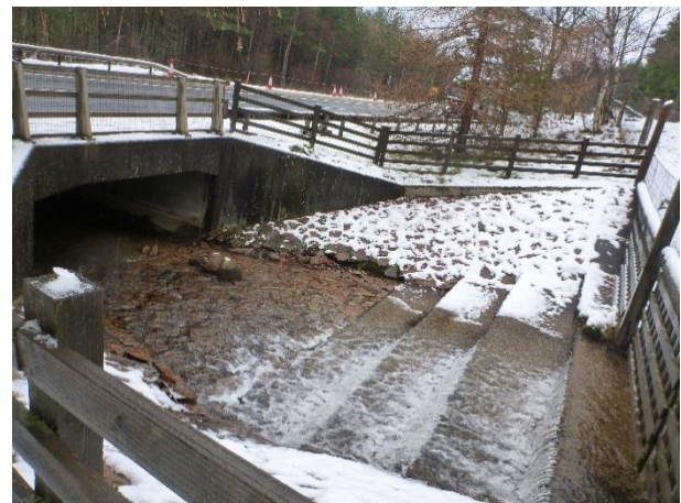
P1040419 – View of existing A9 crossing with concrete stepped cascade leading into culvert (NGR 2857 8095)
