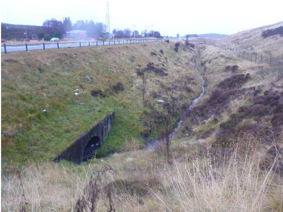
P1040955 – The channel has been realigned and constrained into a narrow artificial valley through a series of culverts (NGR 2836 8256)
