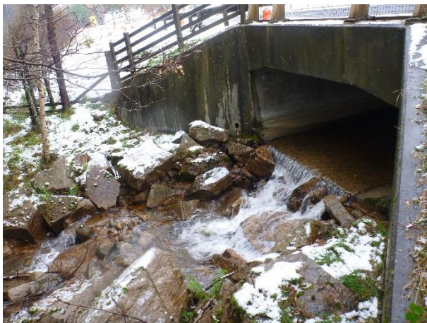
P1040425 – View of culvert outlet with signs of incision downstream and the invert was perched above the channel bed (NGR 2857 8095)
