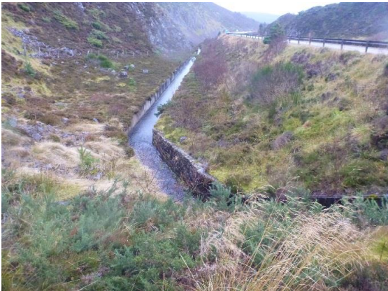
P1040973 – Downstream of the A9 the channel was contained within a concrete lined uniform channel with a steep gradient (NGR 2838 8253)
