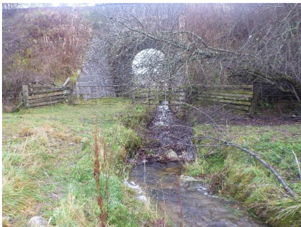
P1040720 – View downstream through the railway arch bridge and straight (and lined) channel (NGR 2911 8185)
