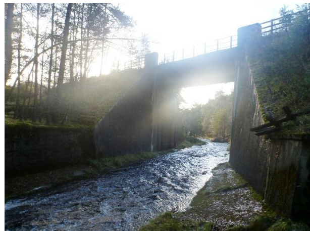
P1040573 – View downstream underneath railway bridge and concrete bed and banks (NGR 2892 8233)
