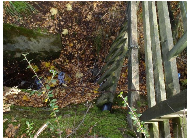
PB110128 – View downstream of structure underneath A9 with minimal flow and a lot of leaf litter (NGR 2904 8167)
