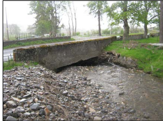
B) Upstream of B9152 – large volume of sediment constricting flow
