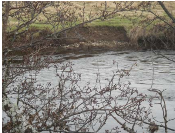
Photograph 11: Erosion bank, of fines over laying gravels. Gravels will be removed at higher flows and the fines will then collapse into channel
