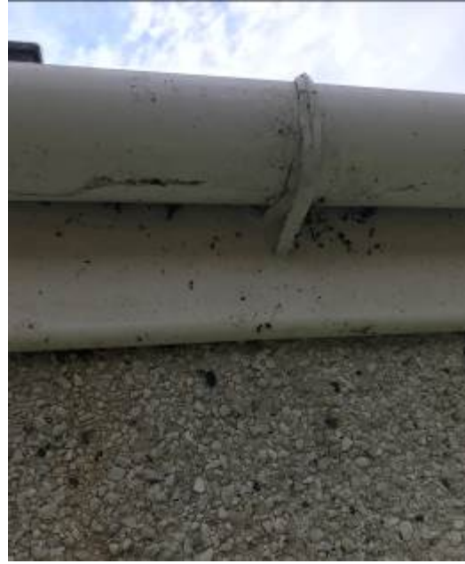
Photograph 12.8.15: Bat droppings between the guttering and fascia board
