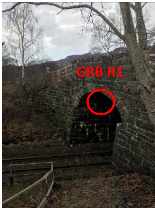
Photograph 12.8.27: Roost with single bat likely underneath the bridge where access was limited.
