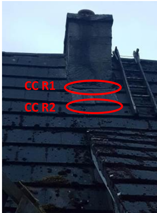
Photograph 12.8.28: Roosts underneath slate roof tiles of Coulintyre Cottage
