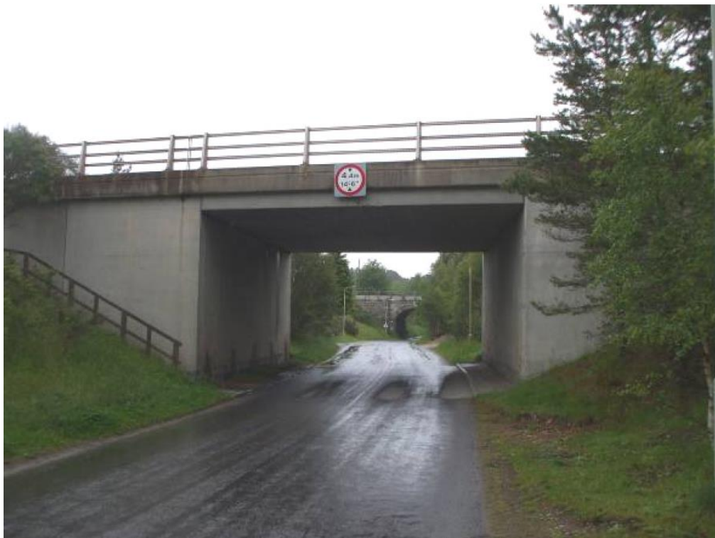
Photograph 2.11.10 Carrbridge Underpass from the west. Note the masonry arch railway bridge in the background.
