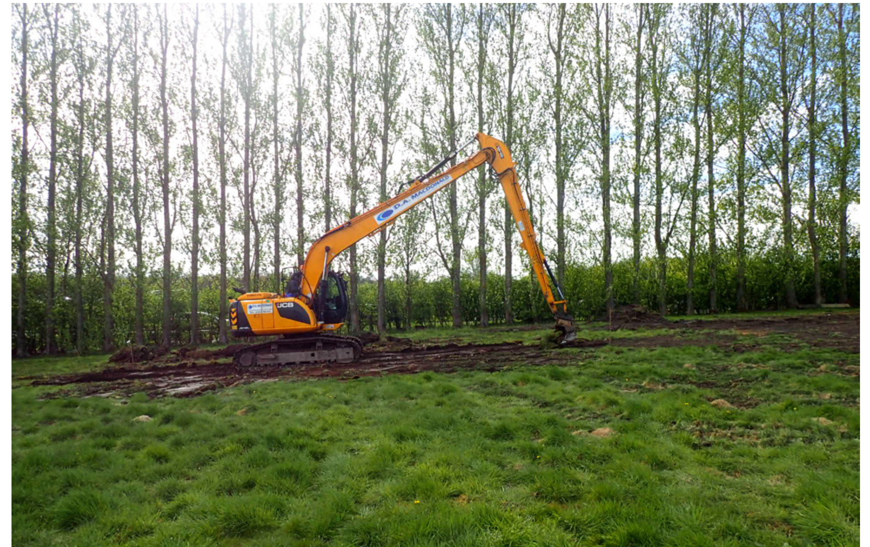
Ground investigation being carried out in a field to the north of Sheriffhall Roundabout
