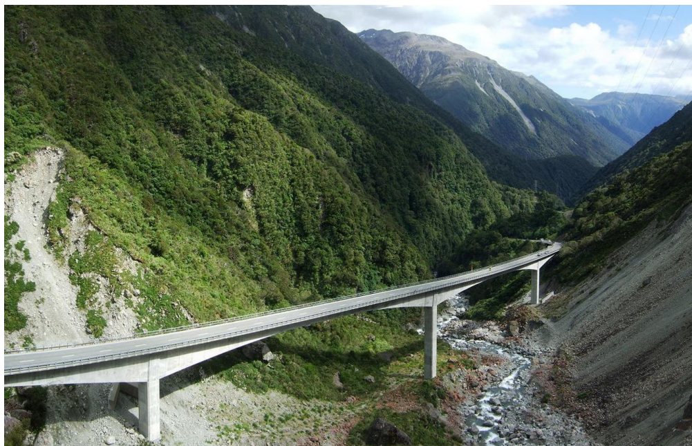
Image C9.30: Example of a large-scale elegant structure – Otira Viaduct, Arthurs Pass, New Zealand / © flickrpd
