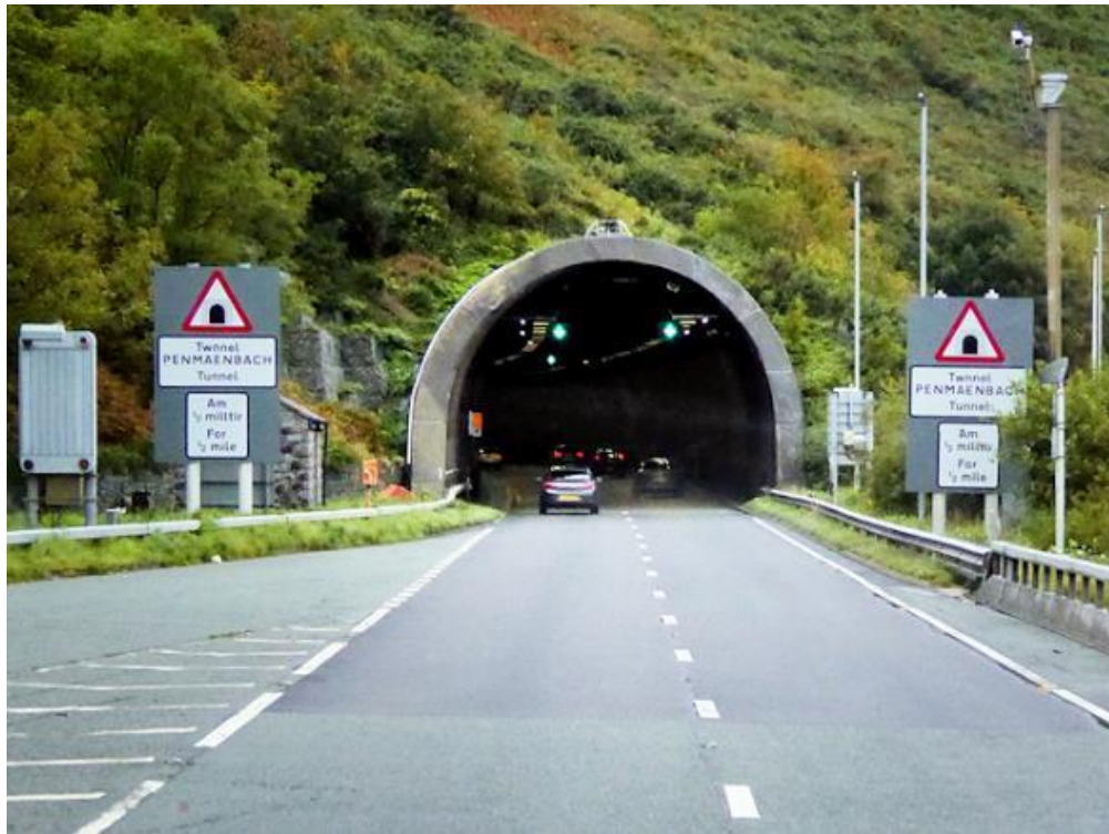
Image C9.34: Example of a tunnel portal - Penmaenbach Tunnel, Eastern Portal, Wales / © David Dixon / cc-by-sa/2.0
