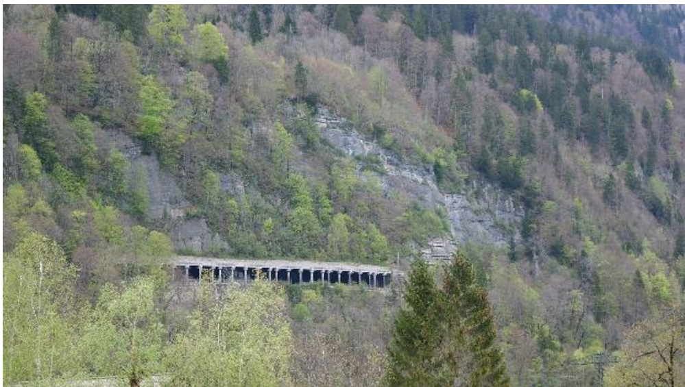
Image C9.23: Example of a canopy structure similar to a debris shelter - Avalanche protection, Austria / © Asumnipal / cc by-sa 4.0
