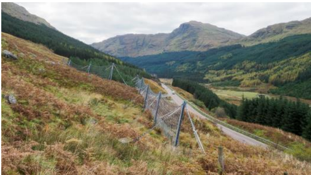
Image C9.20: Landslip defence in Glen Croe / © Trevor Littlewood / cc-by-sa/2.0
