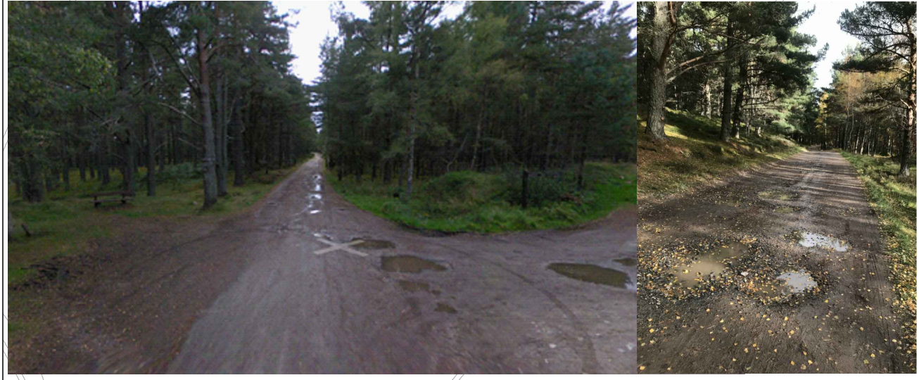
Potholes throughout NCN7 between gated access (Shown On Sheet 3) and Kinchurdy Road
