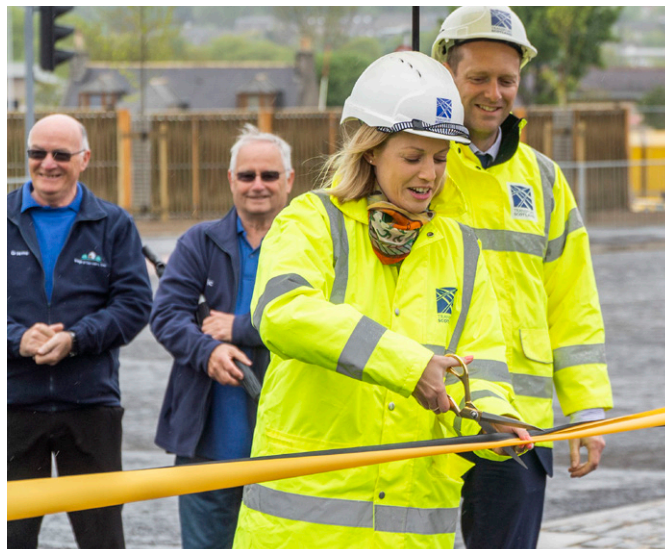
Minister for Transport, Jenny Gilruth cuts the ribbon to officially open the new dual carriageway.
