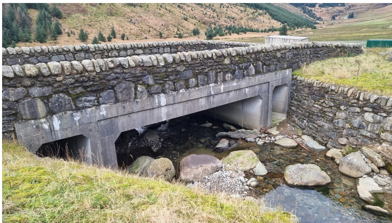
Plate 15.12 OMR crossing of the Croe Water (A83_ML_015_000), looking downstream at the inlet of the structure (Dated: 07 December 2022)
