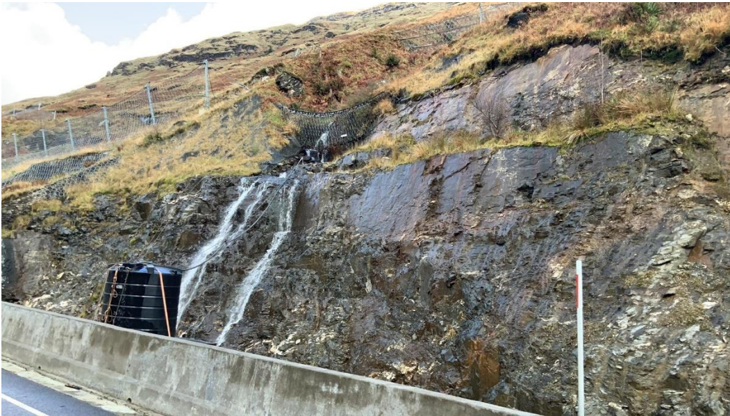
Plate 15.4 Engineered rock slope, adjacent to A83(T) catchpit. Upslope catch fencing across slope and channel. Taken at approximately NGR 223790, 706850 (Dated: November 2022)
