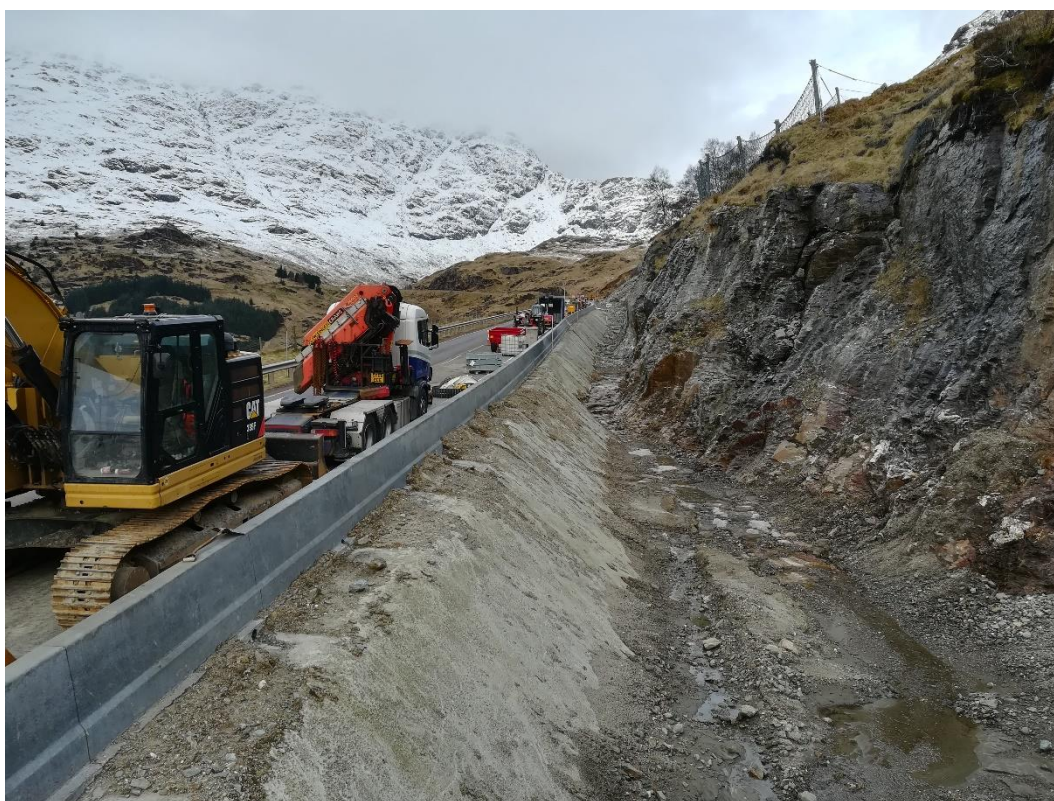
Plate 15.3 Construction of A83(T) catchpit, adjacent to A83(T). Taken at approximately NGR 223790, 706850 (Dated: 31 January 2021)
