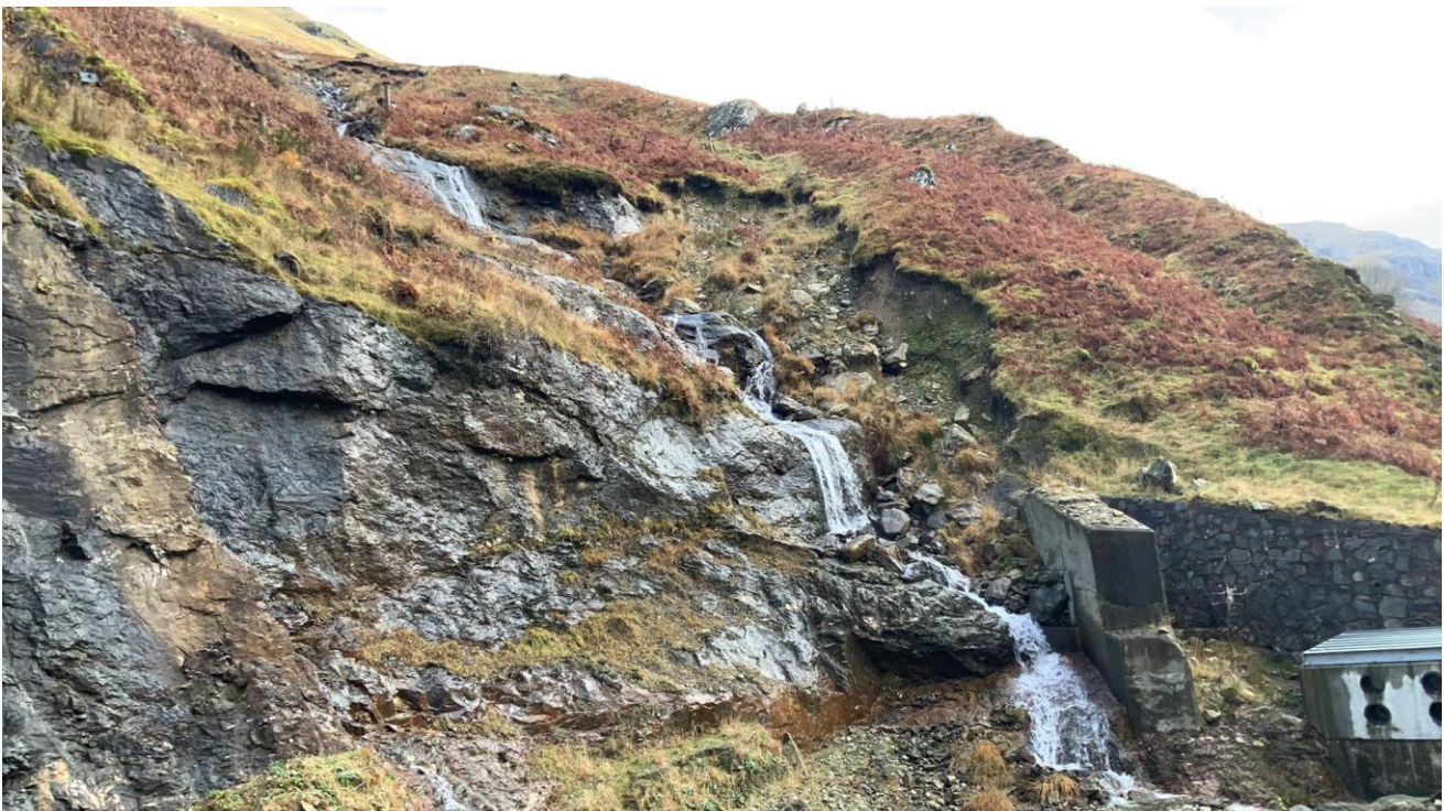
Plate 15.5 Incised channel (A83_ML_024_000) entering catchpit, enclosed inlet to A83(T) culvert on right of image. Taken at approximately NGR 223800, 706830 (Dated: November 2022)
