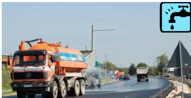
Figure NG 2.3: Watering of surface to avoid sticking of bond coat to tyres
